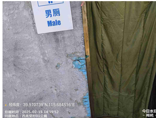
东斋堂村南公厕(内墙面瓷砖破损)T14:19
