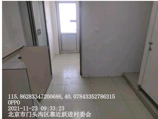
雁翅镇山神庙村公厕（现场检查未见灭火器）T10:16
